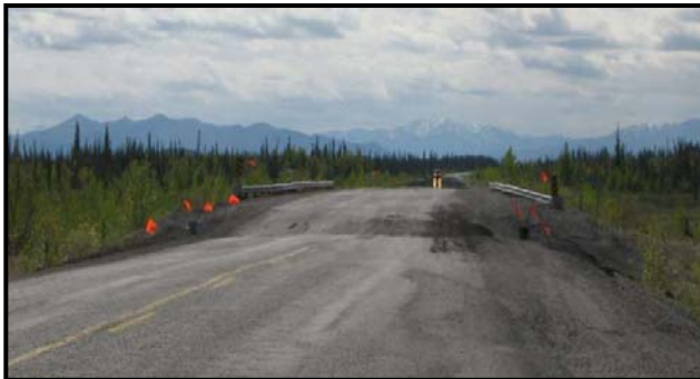
Left: Impacts from thawing permafrost on Alaska Highway north of Beaver Creek (Source: Prof. Billy Connor, University of Alaska Fairbanks 2009, Permafrost and the Alaska Highway) Below: Storm surge undercutting western Alaskan coast (Source: IAWG Final Report)
