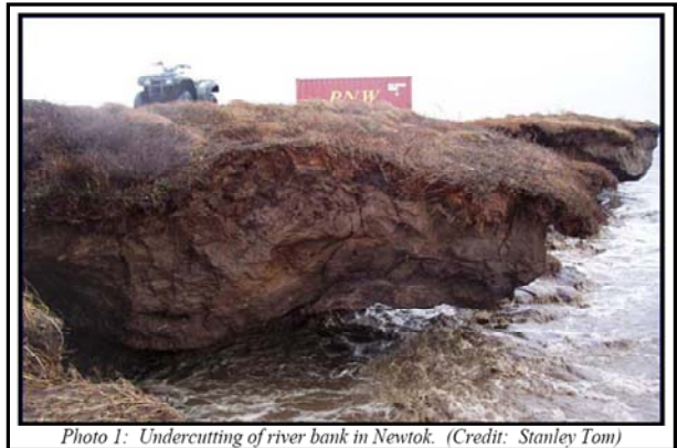
Photo 1: Undercutting of river bank in Newtok. (Credit: Stanley Tom)
